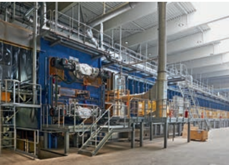
Press discharge end with drive system
