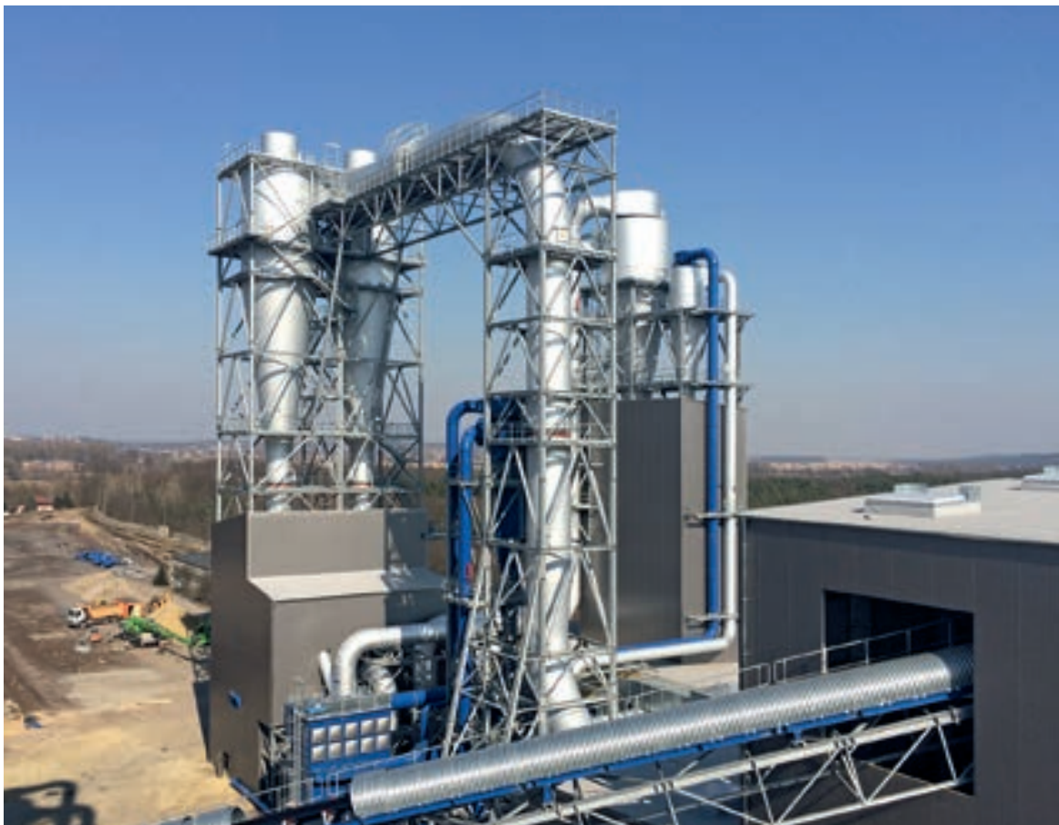
Homanit, Grosno, Poland: Büttner fibre dryer and energy plant for the new MDF plant by Siempelkamp
