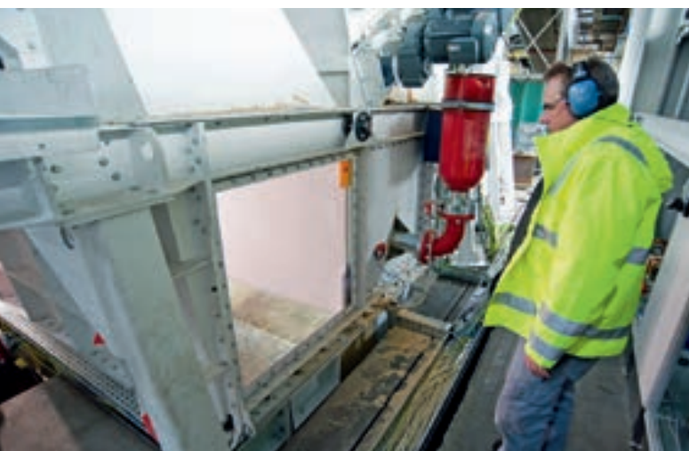
Commissioning in load operation
