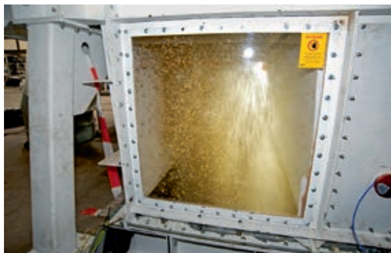
Transport air flow behind Plexiglas
