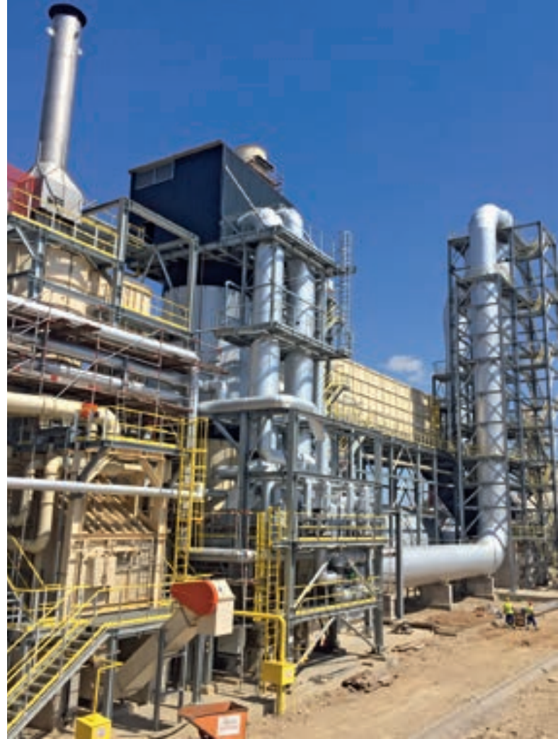
Swiss Krono in Vasarosnameny, Hungary: Büttner energy plant and strand dryer with the new metering bin for wet strands
