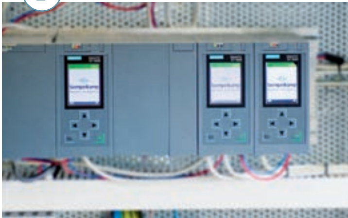
Switch cabinet with control system
